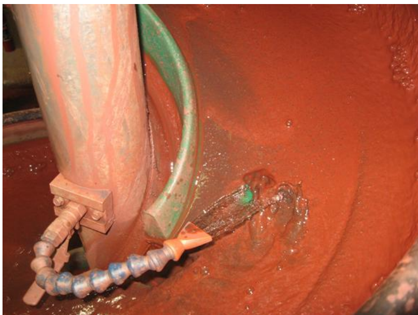
Figure 3 – Wash water setup
